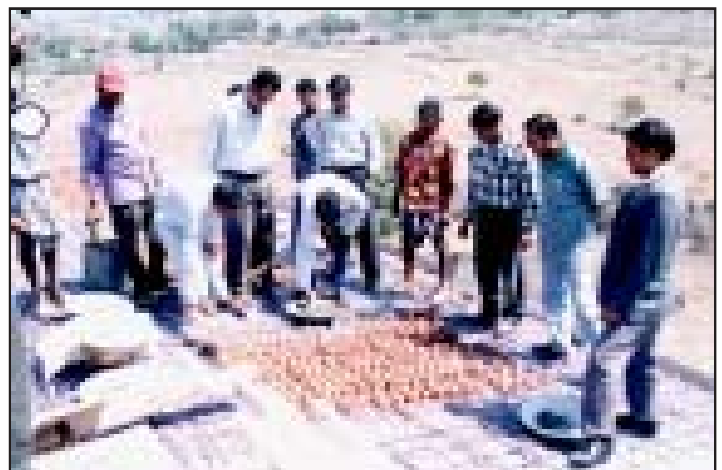
Ingenious cost-cutting methods of building a school roof – Bihar, India. For more on the project on primary education for girls from tribal and minority groups. (see page 5)
